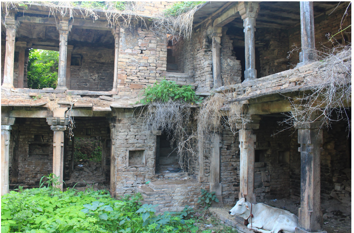
Figure 28 : Structural and architectural depletion at Chaudhari Haveli, Ramnagar
