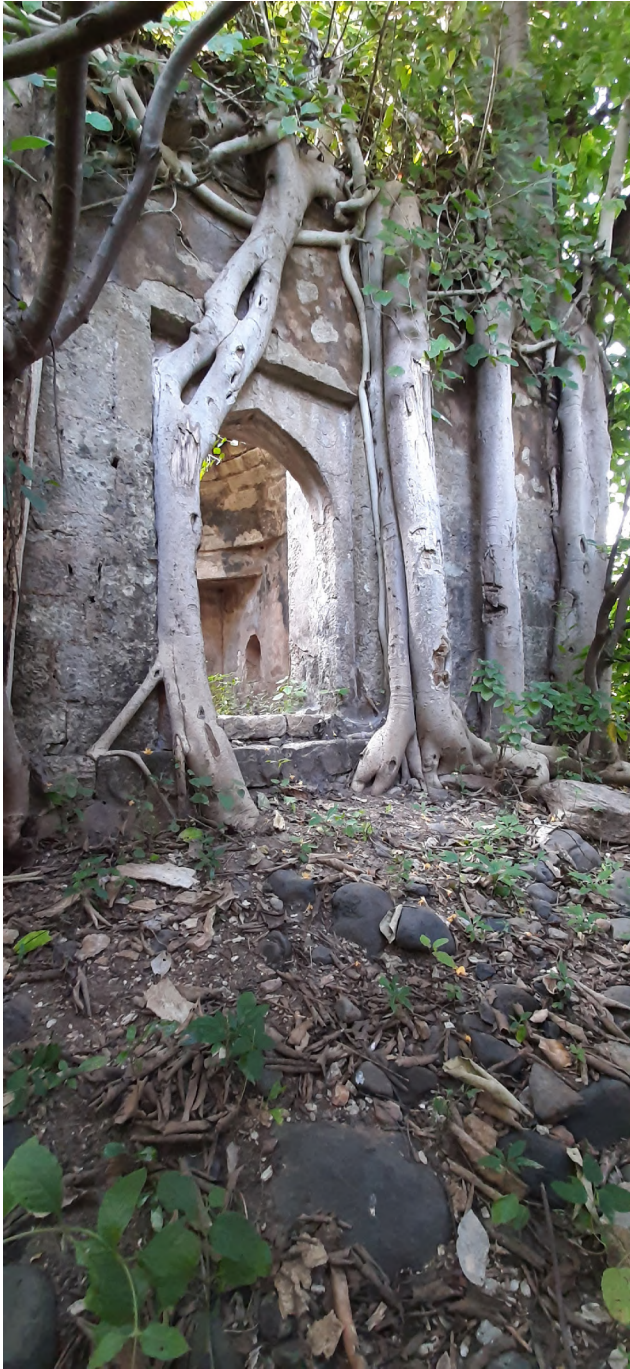
Figure 29 : Vegetation growth damaging the structural integrity, Deogarh
