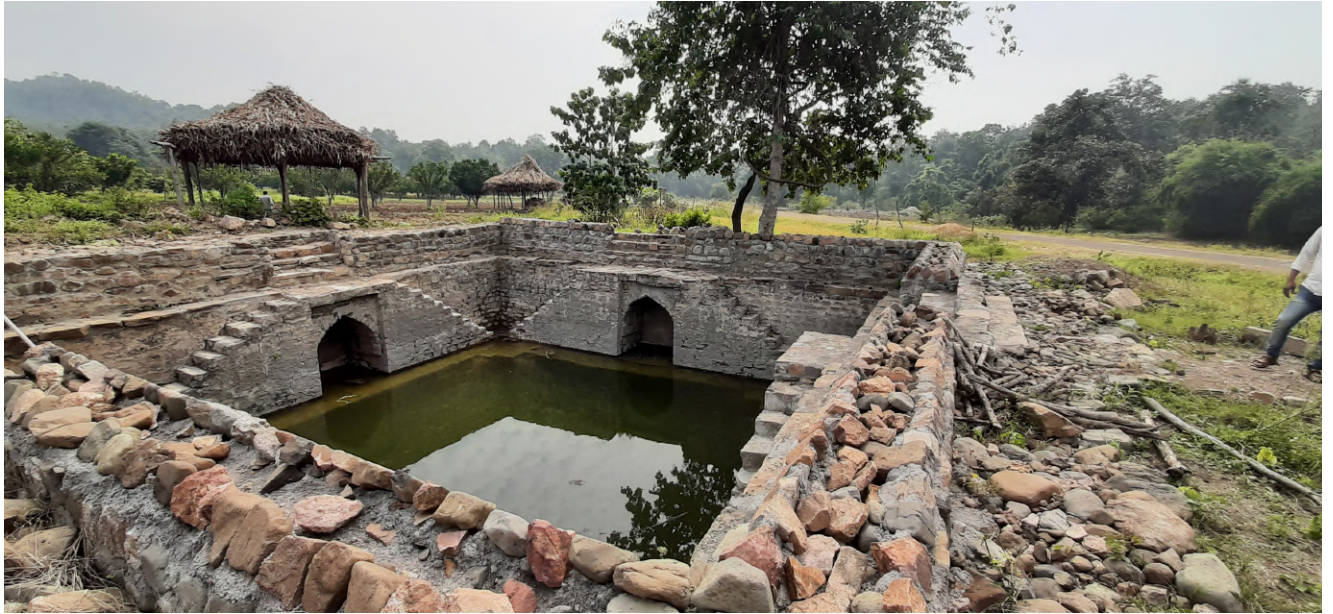
Figure 37 : Dilapidated condition of stepwell in bhajanal farm , Deogarh
