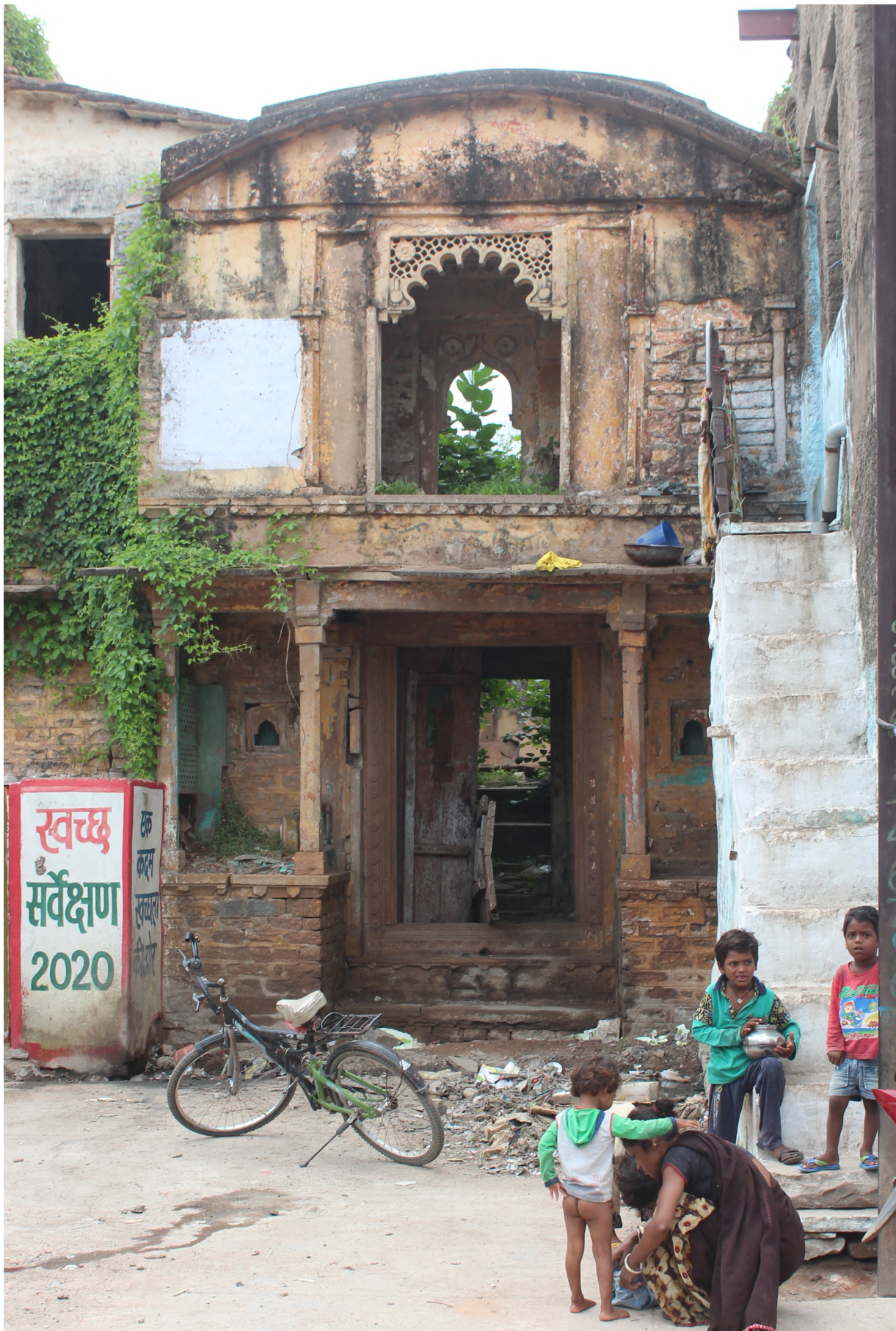
Figure 45 : Abandoned haveli structure, Chanderi
