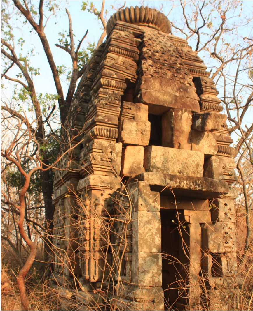
Figure 34 : Isolated and damaged heritage structure, Bandhavgad
